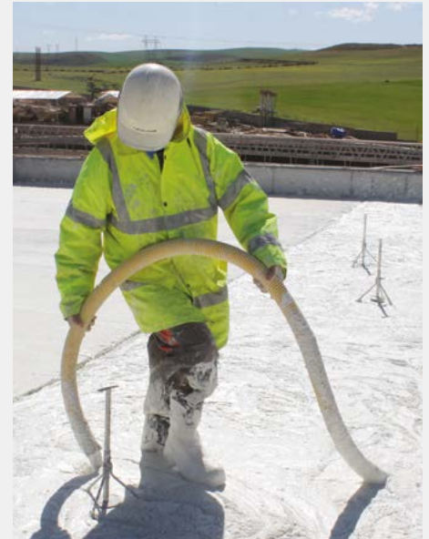
Algeria AIRIUM project.
